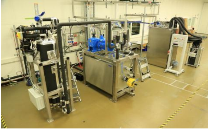
Figure 1: 15kW TIF plant at CERN
