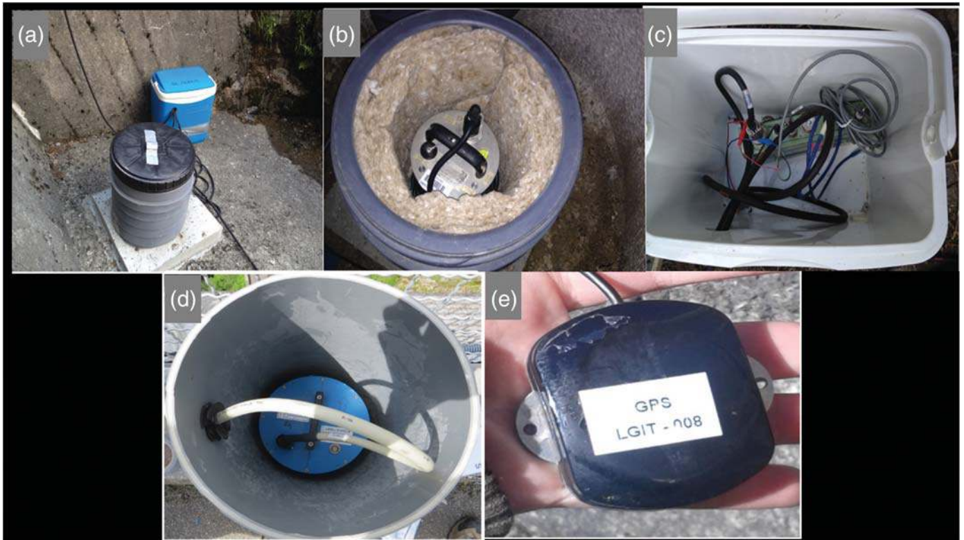
Figure 3. Station details. (a) Final installation of a station along the dam–rock interface. (b) The gray plastic cylinder sealed within the concrete slab contains the CMG40T sensor surrounded by a thermal isolation wool, and (c) the blue plastic device contains the Nanometrics Taurus digitizer and its cables. (d) The Lennartz-3D-5s sensors installed on the crest of the dam use smaller plastic cylinders and no thermal isolation. (e) A Global Positioning System (GPS) receiver is added to each station for time synchronization.
