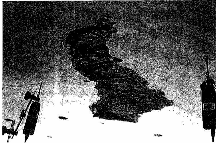
Fig. 14 – Damage pattern on the sub-face of the slab.
